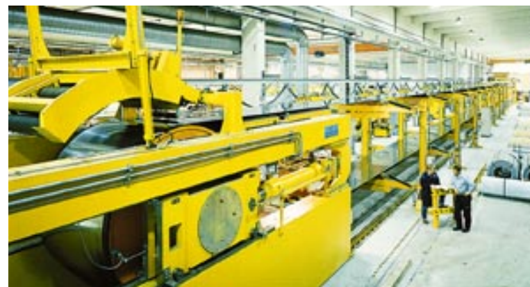
A NEW LEVELING LINE FOR STRIP STEEL WAS INSTALLED DURING THE YEAR IN SANDVIKEN.
