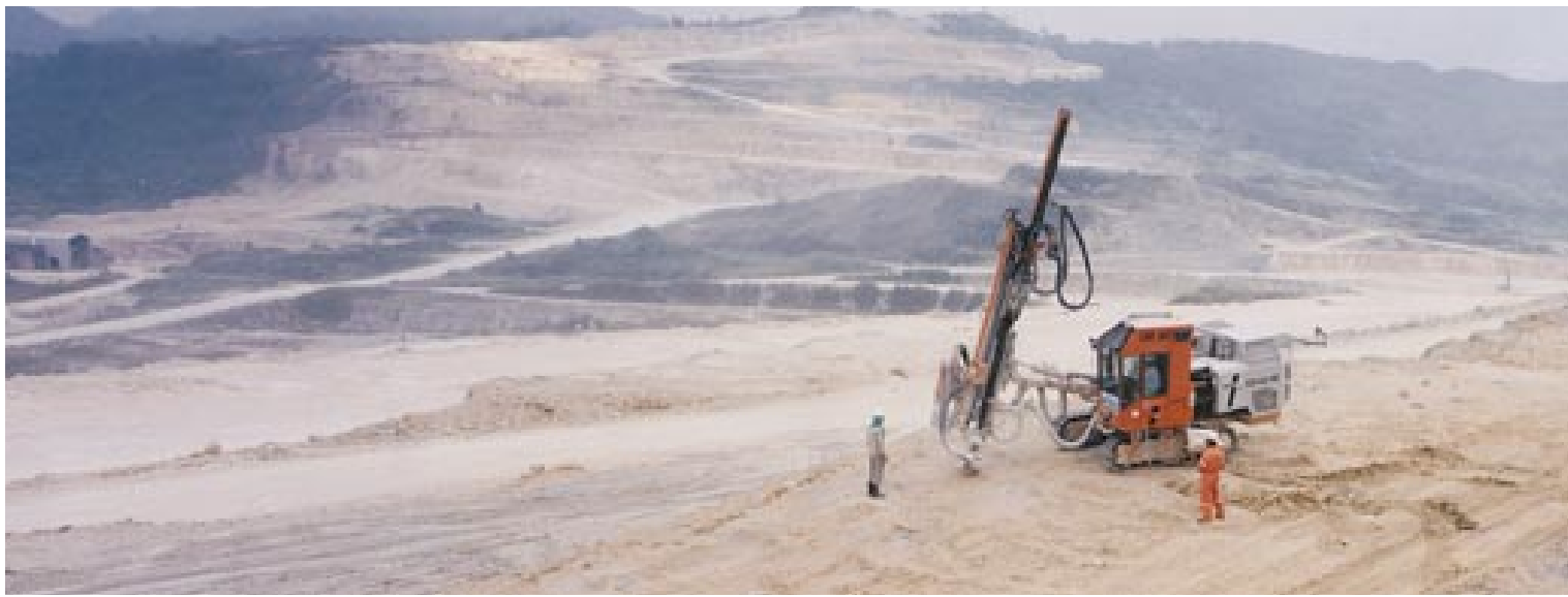
TAMROCK IS INVOLVED IN COMPREHENSIVE INFRASTRUCTURE PROJECTS IN ALL PARTS OF THE WORLD.
